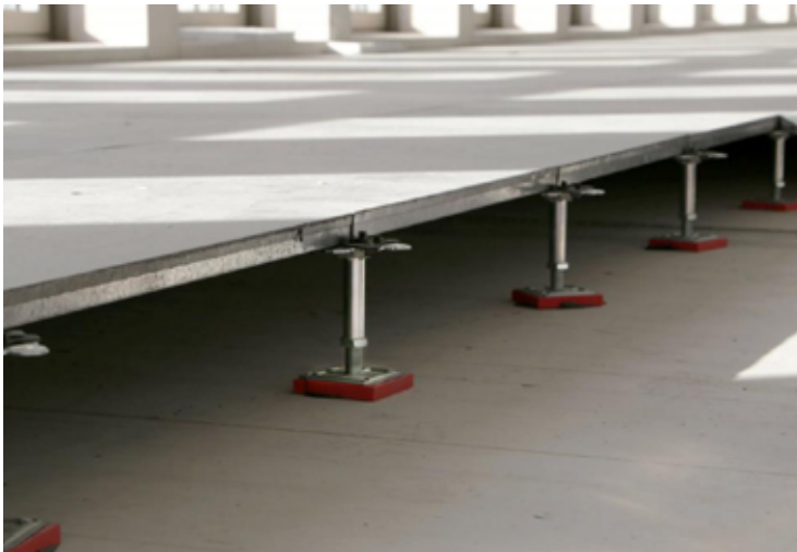
Reuse of raised access floor slabs with new jacks © Mobius - Marie Moroté
