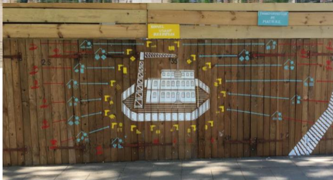
Fresco on the site fence describing the project's reuse approach. Crédits : Bellastock
